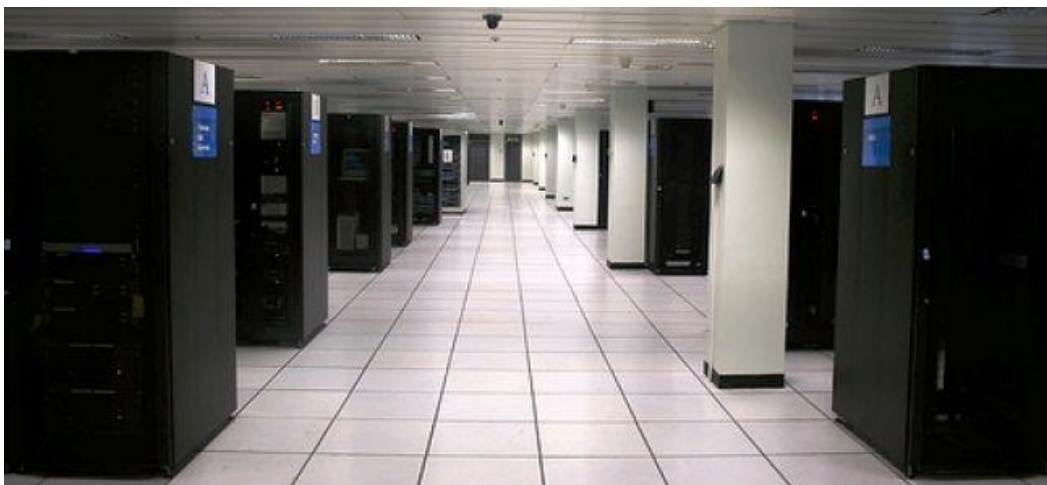
Gambar 1 Ruang Data Center
